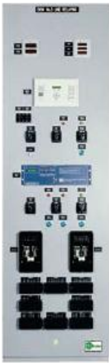
Line Breaker Panel
