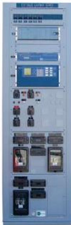
Line Breaker Panel
